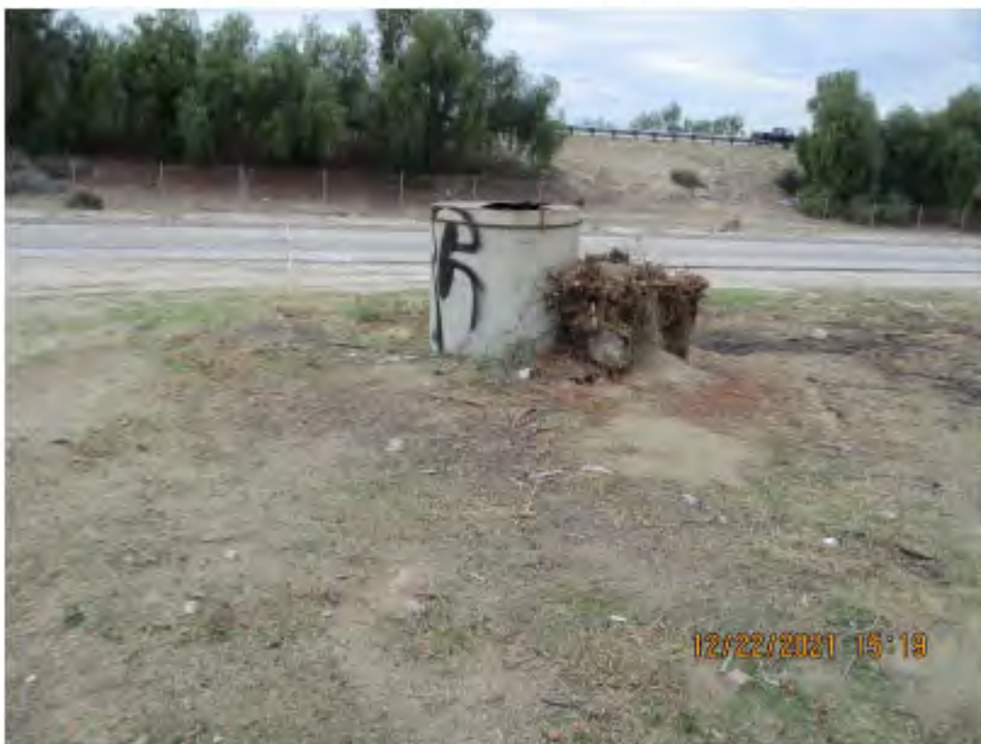
Photo #12 – west view of an irrigation valve riser at the northwest corner of the subject property. Riser is currently filled with trash. 210 Freeway visible in background.
