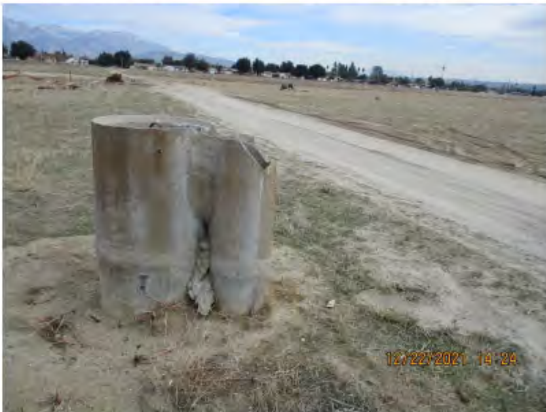
Photo #14 – easterly view of irrigation valve riser near the northeastern portion of the subject property. Irrigation line may trend east west (See Photo #12).
