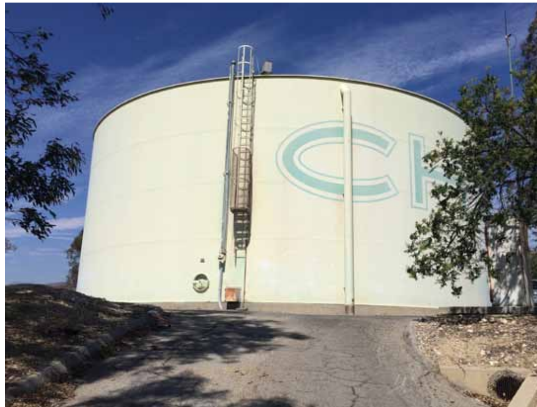
The Crafton Hills Reservoir stores treated water for future use.
