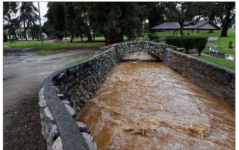
Stormwater flows through the Zanja as it passes through Sylvan Park.
