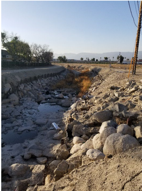
Photograph 1. Looking Northwest at Mission Zanja Channel. Note soft bottom and sides with rip rap are currently in place for stabilization.
