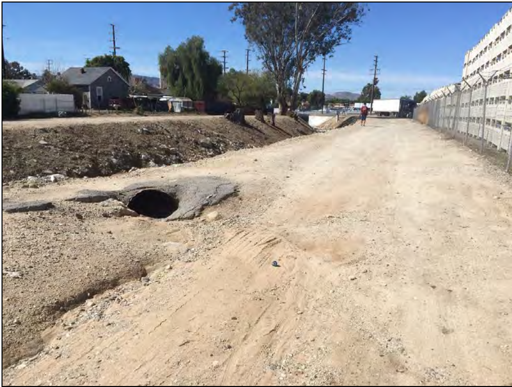
Photo 7: Western terminus of erosional feature and three-foot wide culvert that conveys stormwater runoff into Zanja; facing west.
