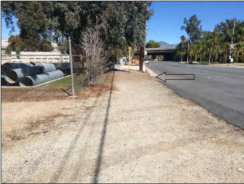
Photo 9: View of starting point of erosional feature along the road edge of Church Street (arrow); facing north.
