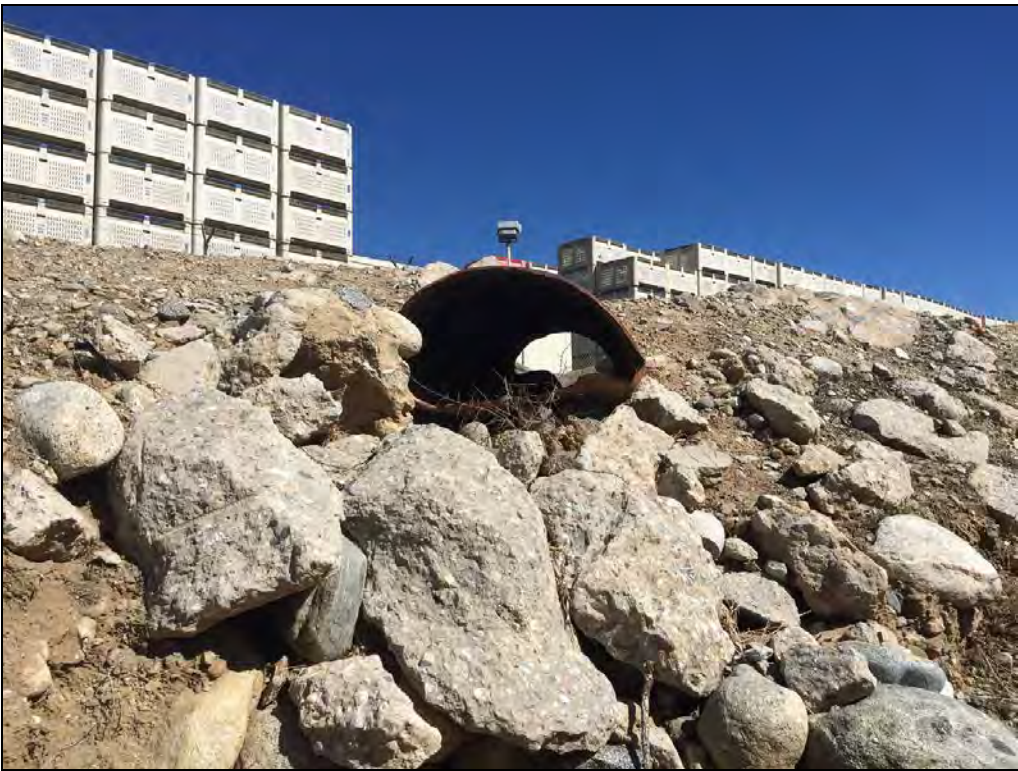
Photo 6: Three-foot wide culvert that conveys stormwater runoff from Church Street into Zanja; facing north.
