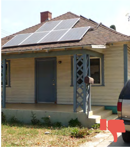
Avoid installing solar panels at the front of a roof.
