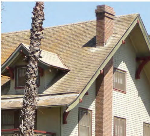
Inspect seismically vulnerable historic components, such as chimneys, to ensure they are structurally sound.
