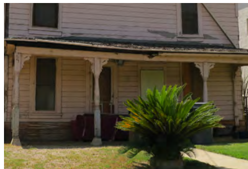
Weakened or sagging features, such as this porch roof, suggest the need for structural repair.
