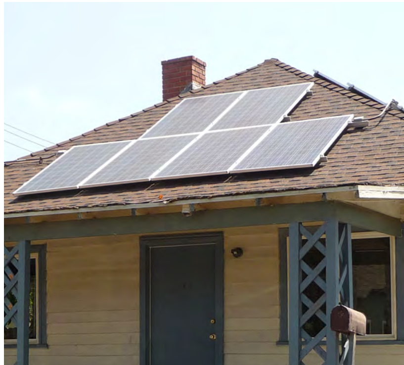
Solar panels on a composition shingle roof.
