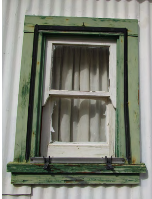
Weathered and racked window needing repair.
