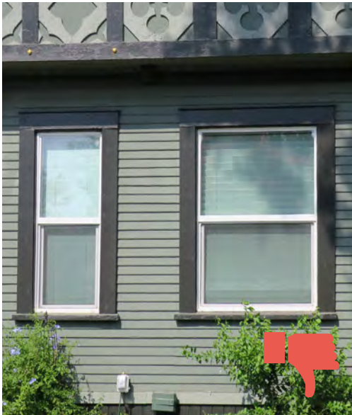
Avoid replacing windows with stock items that are incompatible with the historic materials or colors of the building.
