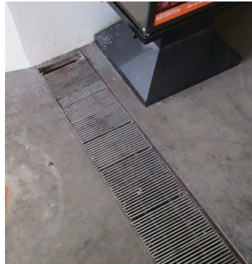
Drain with uneven grate panels.
