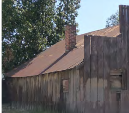
Corroded and warped corrugated metal roof.
