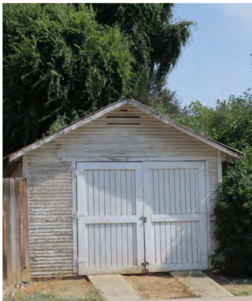
Routine maintenance, such as painting, is important to the preservation of a historic ancillary structure.
