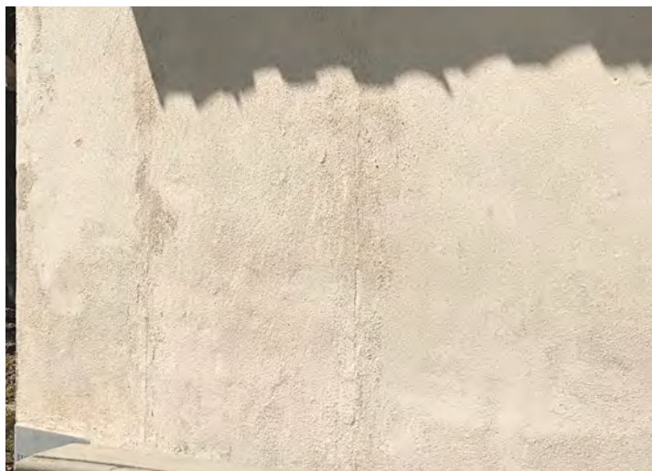
Incompatible stucco at an infilled door.
