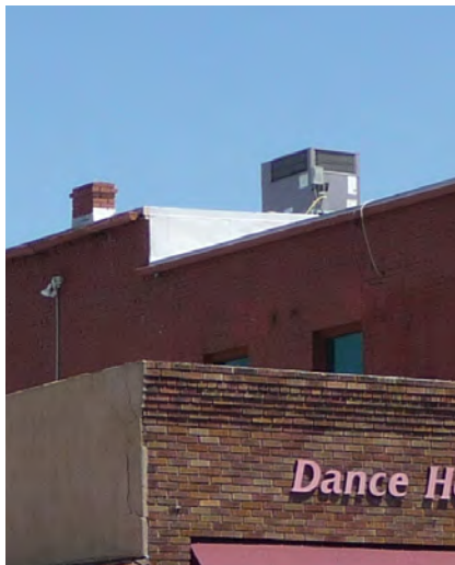
HVAC equipment atop a commercial building.
