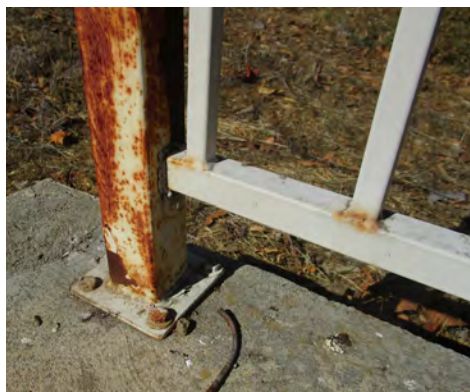
Example of rust at a painted metal fence.
