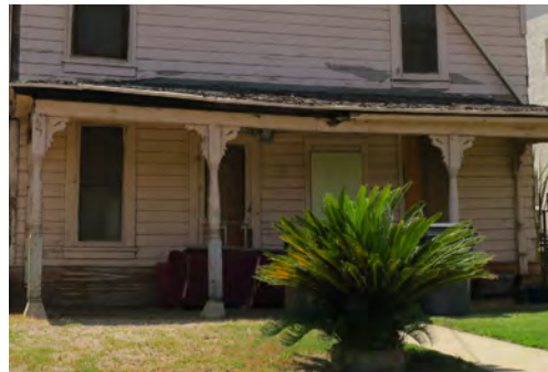
Weakened or sagging features, such as this porch roof, suggest the need for structural repair.
