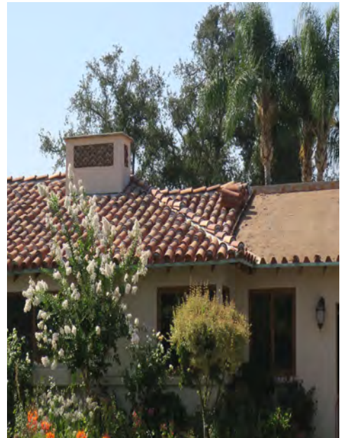
New roof tiles or shingles should match the material, size, profile, and color of the historic roof as closely as possible.
