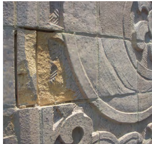
Damaged terra cotta detail.
