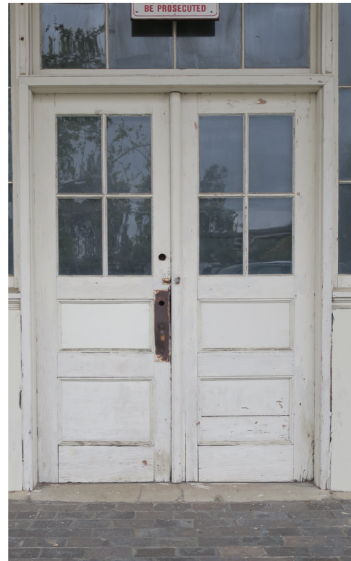
Weathered doors with corroded and missing hardware.
