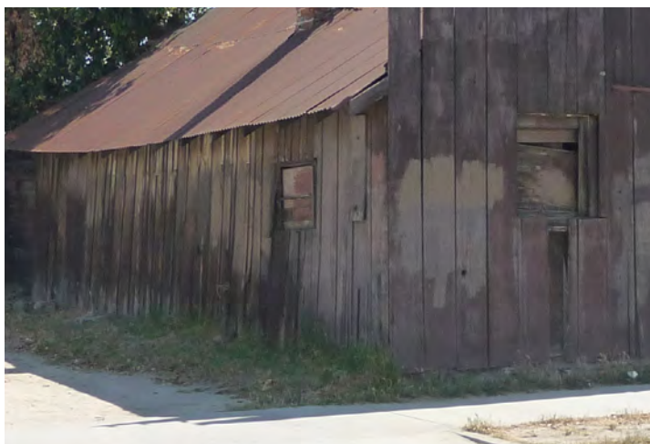
Direct contact with the ground can lead to wood decay.
