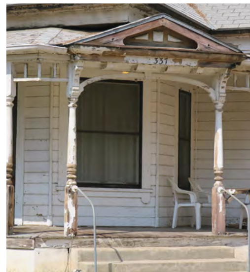
Deteriorated woodwork at a porch.
