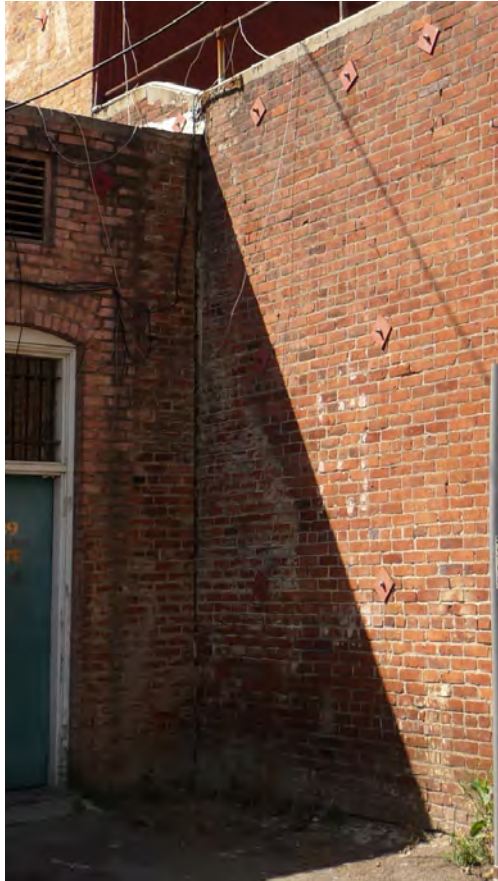
Efflorescence on a historic brick wall.
