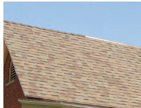
Reattach or replace loose or missing shingles.
