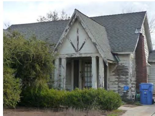
Poorly maintained wood cladding and trim.
