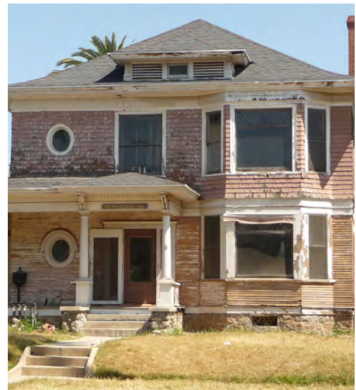
Weathered paint on exterior woodwork.
