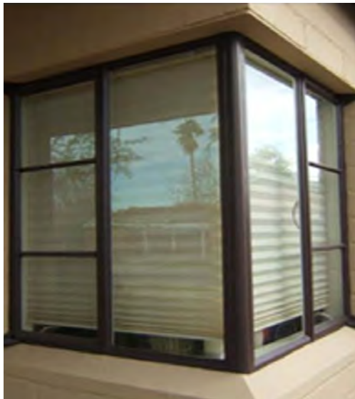
Retrofitting original windows with historically compatible, low-e glass is a way to achieve greater energy efficiency. (Photo, City of Phoenix Planning and Development Department, Historic Preservation Office, 2018.)
