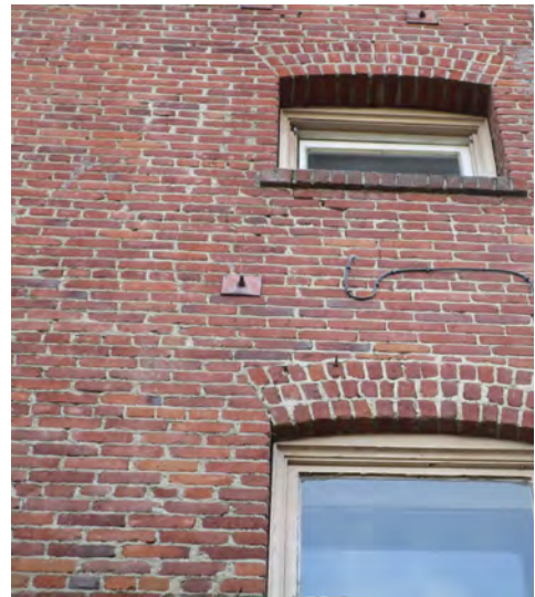
An example of seismic anchor plates that blend in with the surrounding brick.
