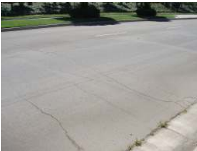
Barton Road west of Lakeside Avenue (PCI = 70). Moderately weathered road, little or no patchwork. Some minor transverse cracks.
