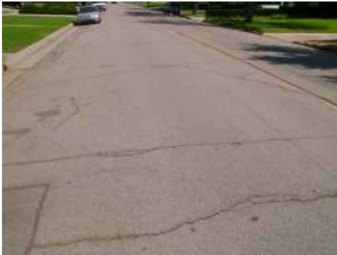
Palm Avenue near San Jacinto Street (PCI = 66). Weathered, medium severity transverse cracking with some edge cracks.
