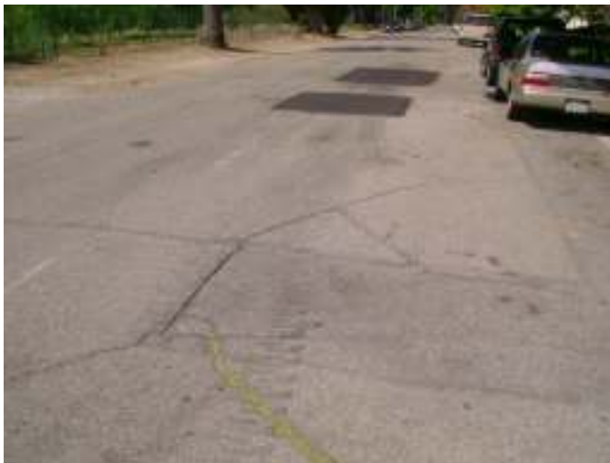
Stillman Avenue west of Judson (PCI = 66). Some weathering, medium severity transverse cracking, low-severity patch work. Note the different distresses on two roads rated with a PCI of 66.
