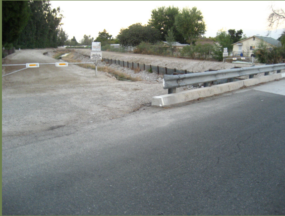
Zanja Creek at New Jersey St. facing west
