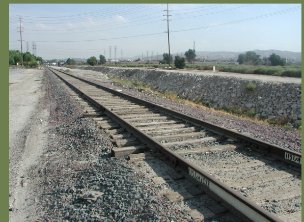
Magnolia Channel and tracks at Mountain View Ave. with maintenance road on south bank facing east
