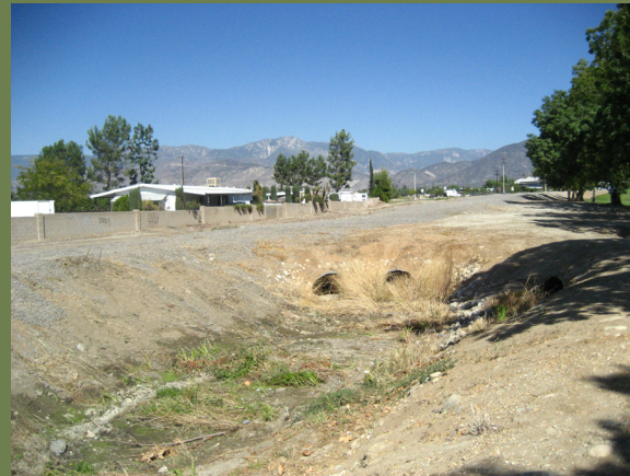
Drainage outlets along drainage channel north of Crafton Park creating erosion issues on existing maintenance road - facing east toward Wabash Ave.
