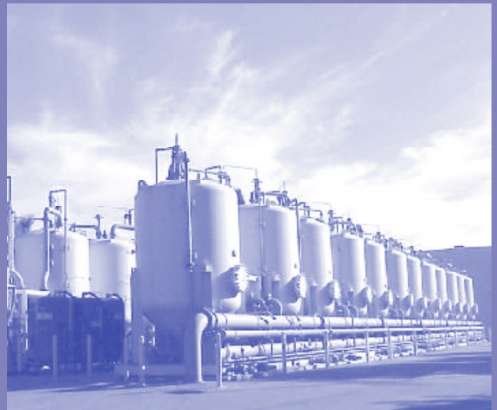
Treatment facilities like this help to ensure high quality water is delivered to all of our customers
