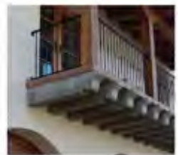
WOOD BEAM BALCONY
