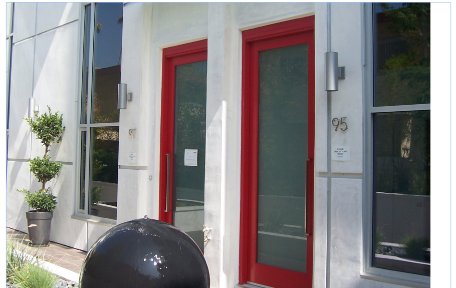
Lamps, address signs, and door hardware are consistent with each other and the building.
