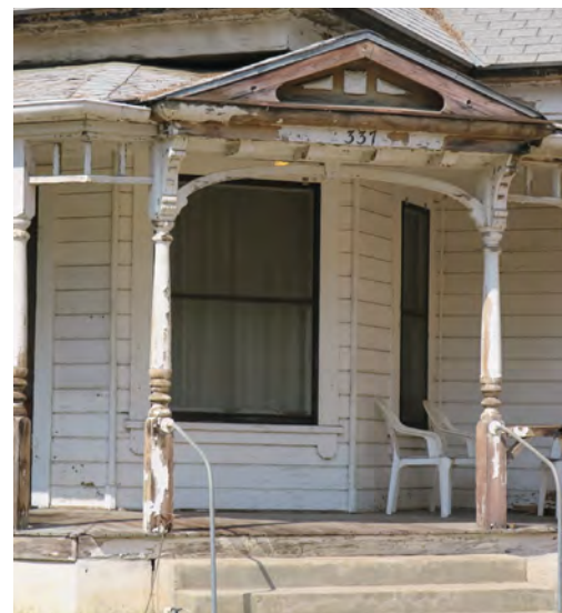
Deteriorated woodwork at a porch.
