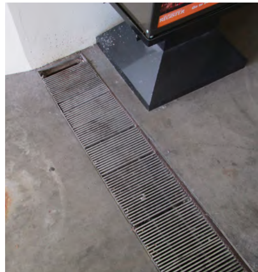
Drain with uneven grate panels.
