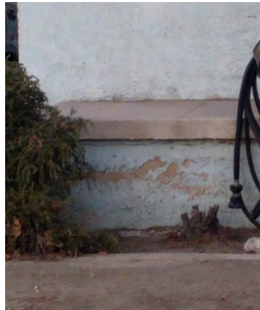
Weathered stucco at a porch.
