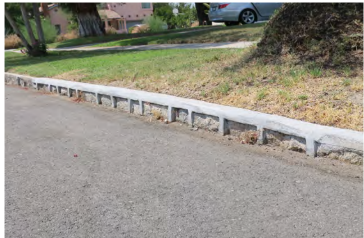
Inappropriate concrete repairs to cut stone curbing.
