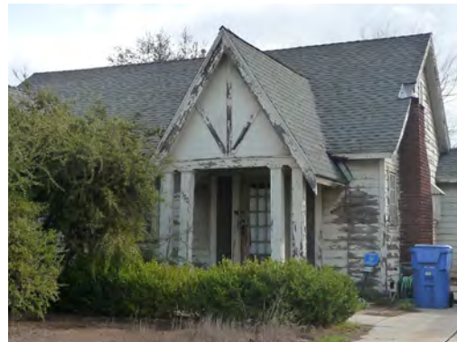
Poorly maintained wood cladding and trim.
