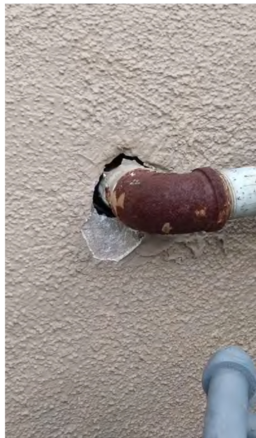
Void and spalling around stucco wall pipe intrusion.
