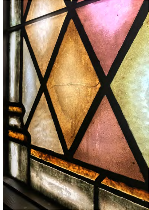
Cracked glazing in a stained glass window.
