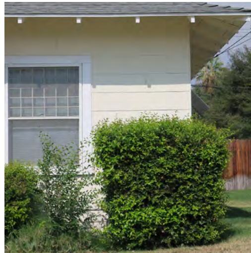
Avoid covering or replacing wood siding with synthetic siding.
