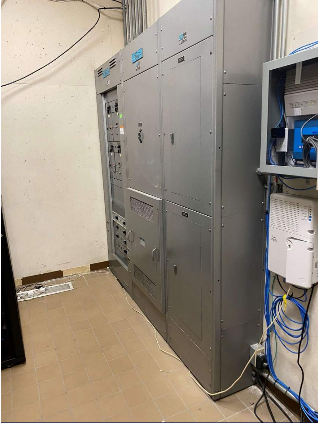
Figure 26 MCC and Communications Equipment
