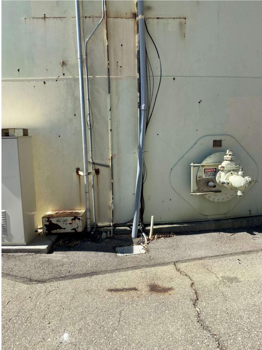
Figure 41 Signs of Aging and Corrosion are Evident
