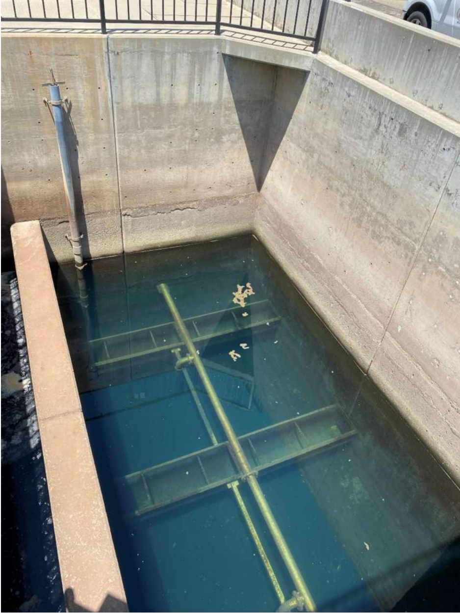
Figure 6 Hinckley WTP Filters
