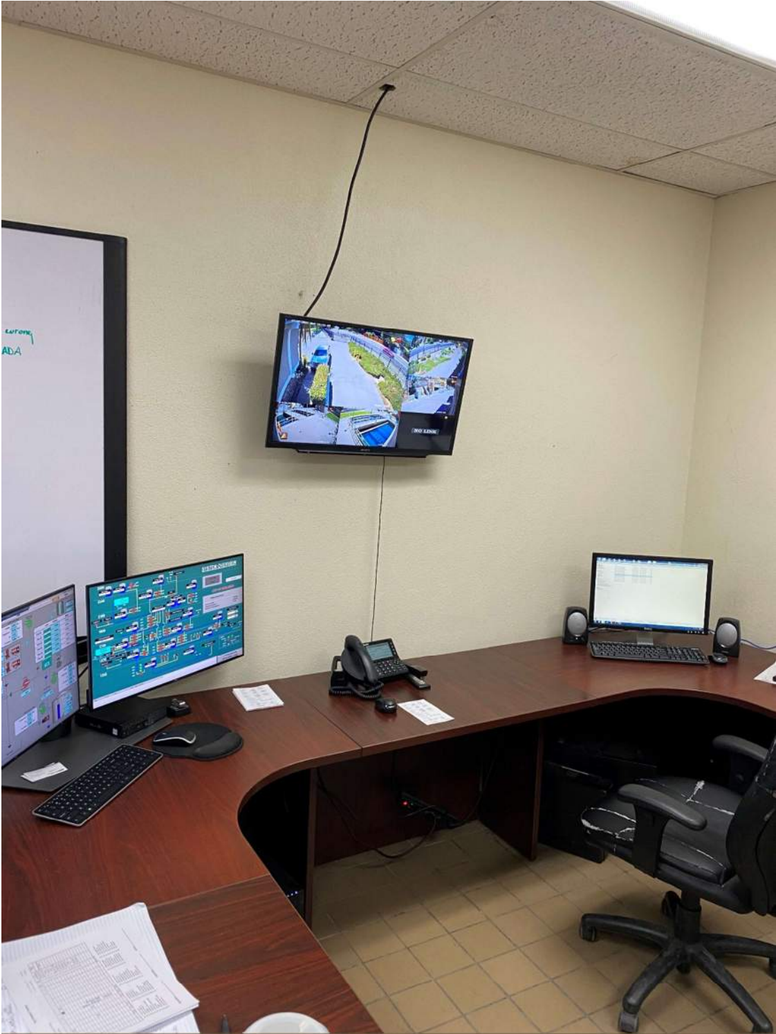
Figure 27 Control Room-Excellent Working Condition
