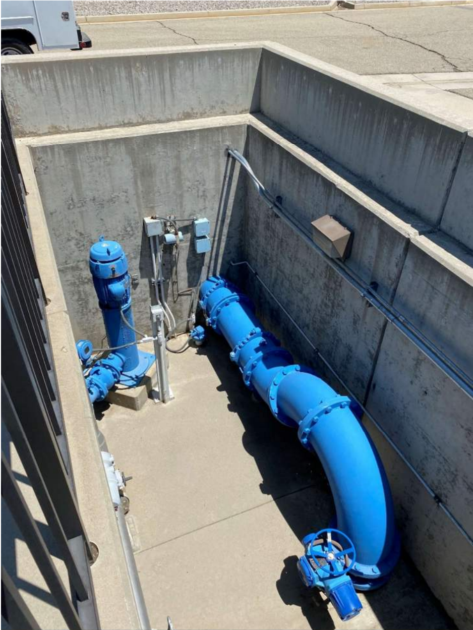
Figure 5 Hinckley WTP Flocculation and Sedimentation Basin Inlet
