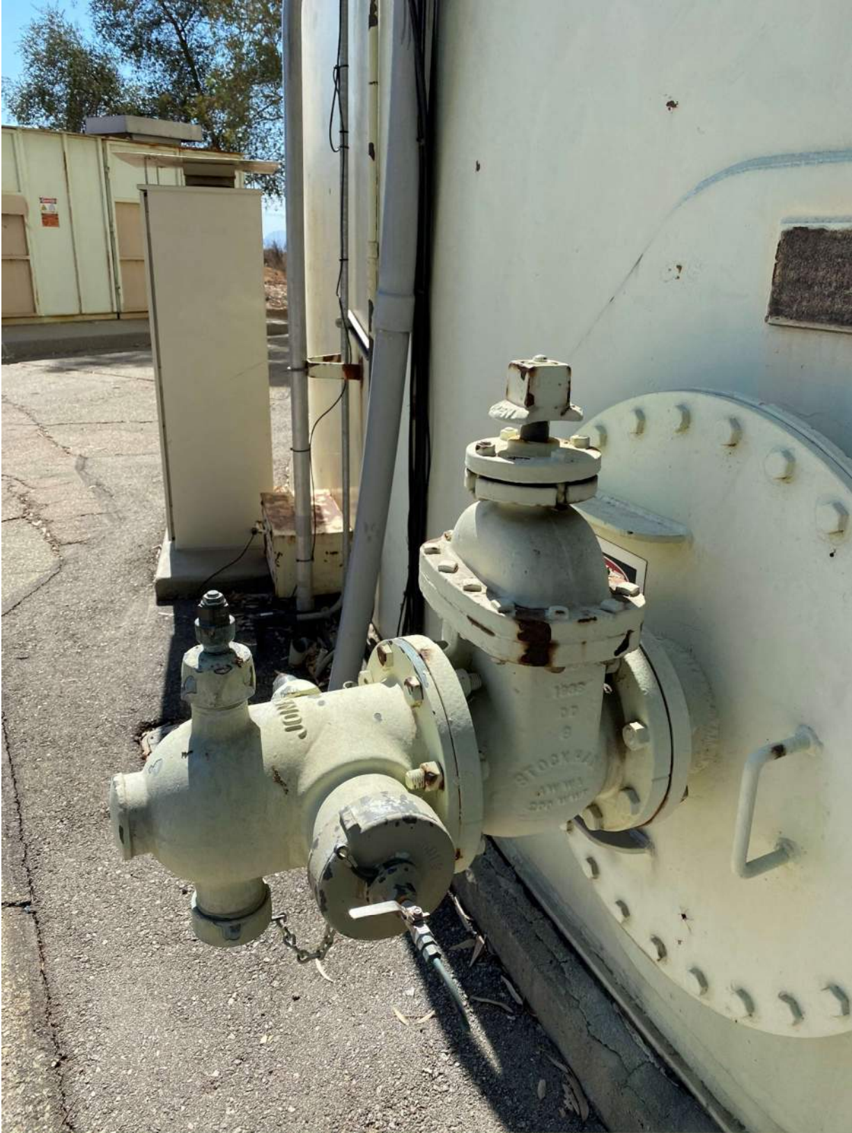
Figure 48 Access Manhole Valve is Corroded
