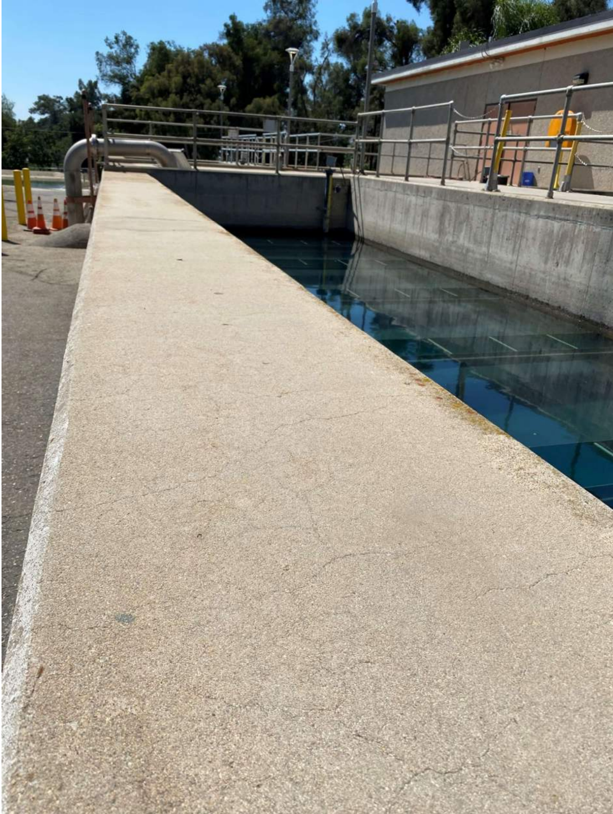
Figure 38 Filter Equipment (Seems to be an Excellent Working Condition)
