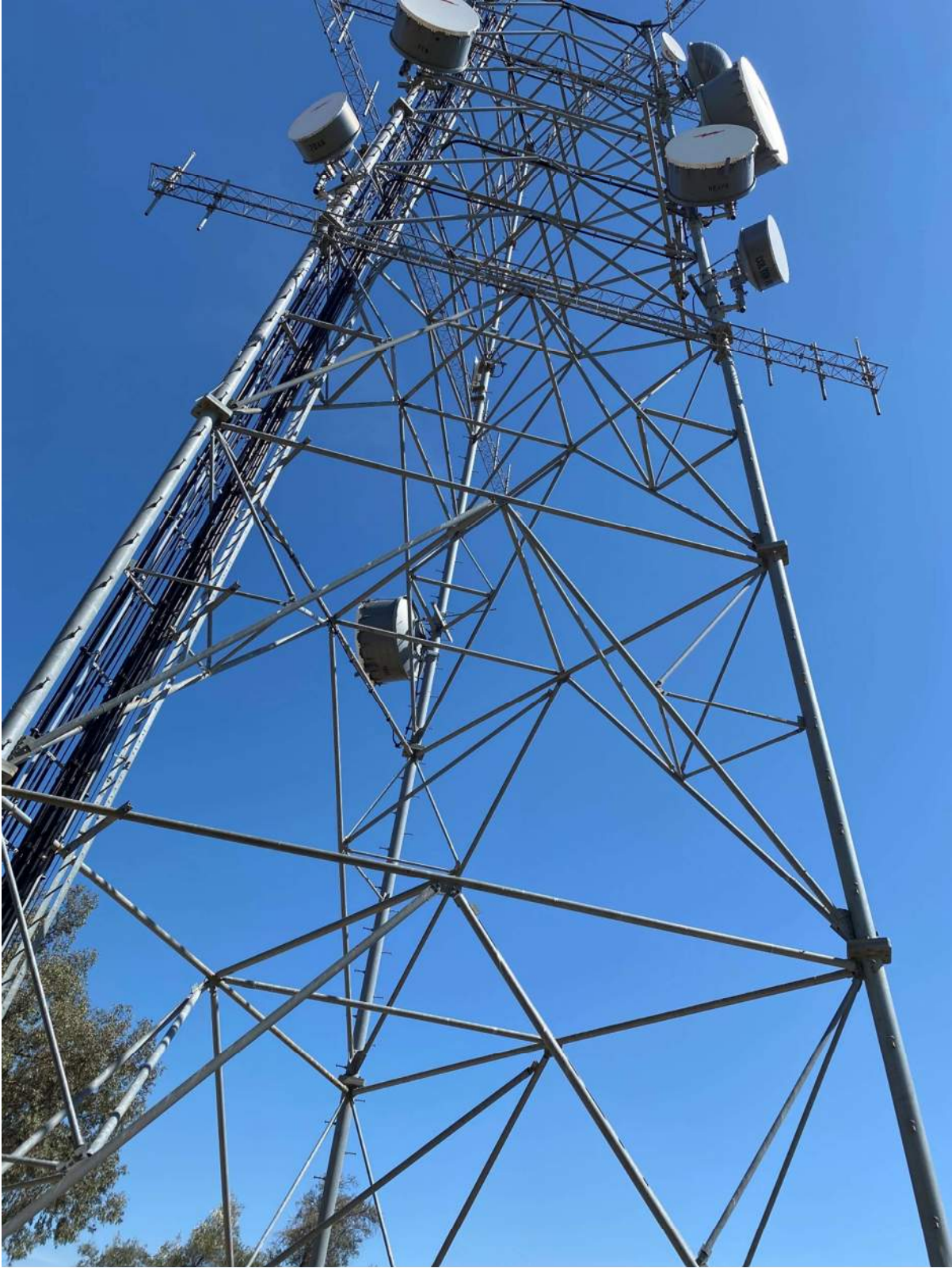
Figure 42 Communication Antenna of Service Provider Erected Onsite
