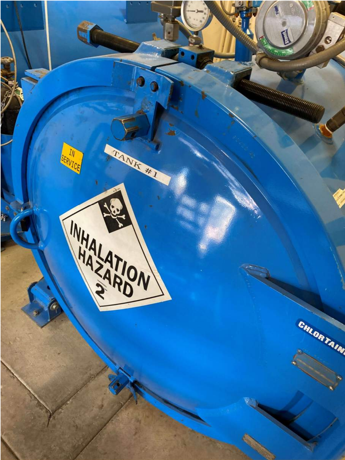
Figure 30 Safety Enclosure of the Chlorinators
