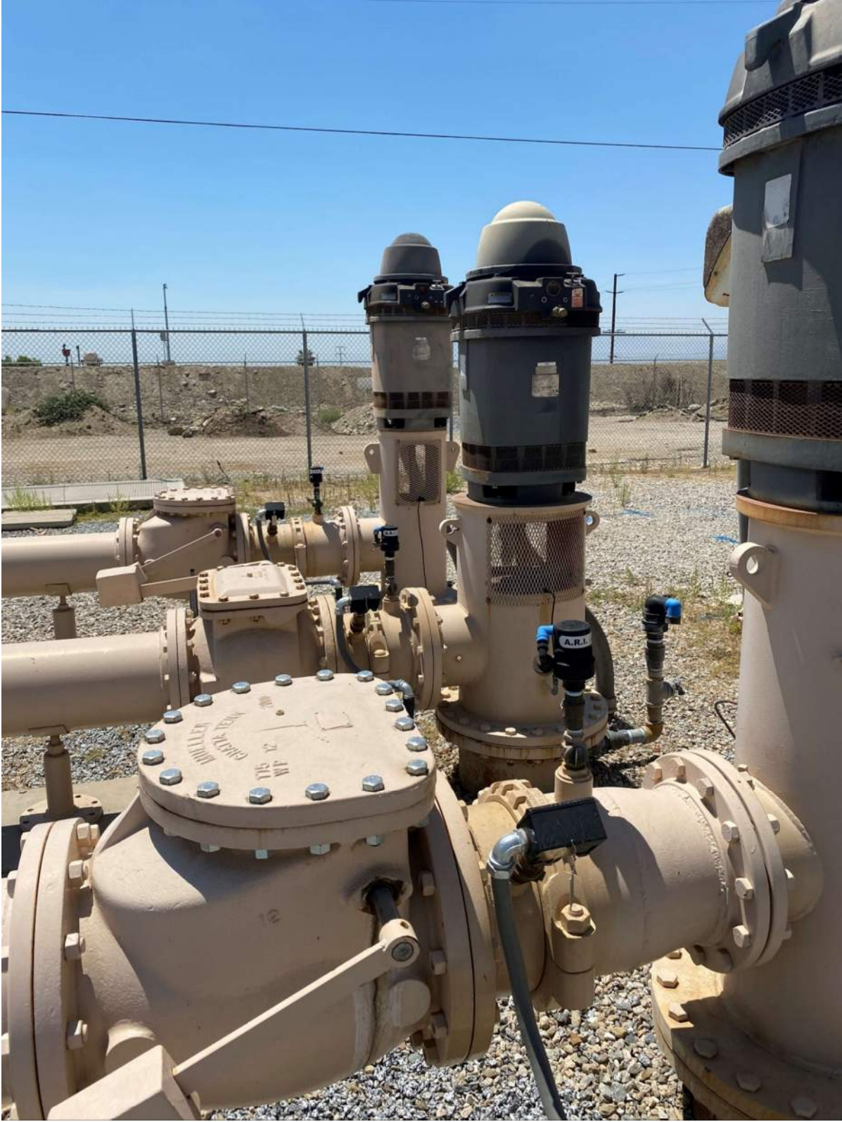
Figure 23 Booster PS Discharge Valves and Pressure Gauges
