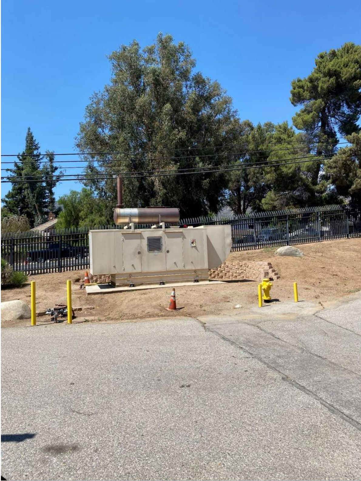
Figure 33 Standby Diesel Generator Set
