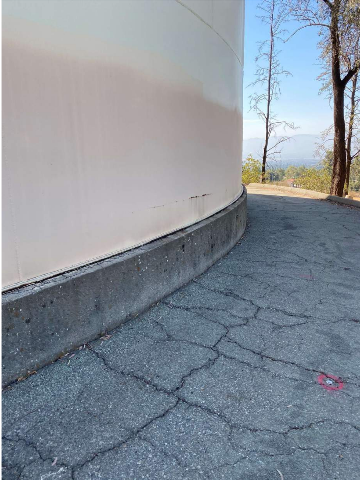
Figure 46 Reservoir Base (surrounding asphalt is cracking and evidence of deterioration)
