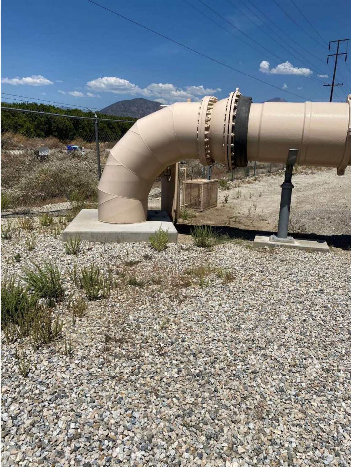
Figure 16 Agate Reservoir Seismic Expansion Unit Supported Off the Concrete Slab
