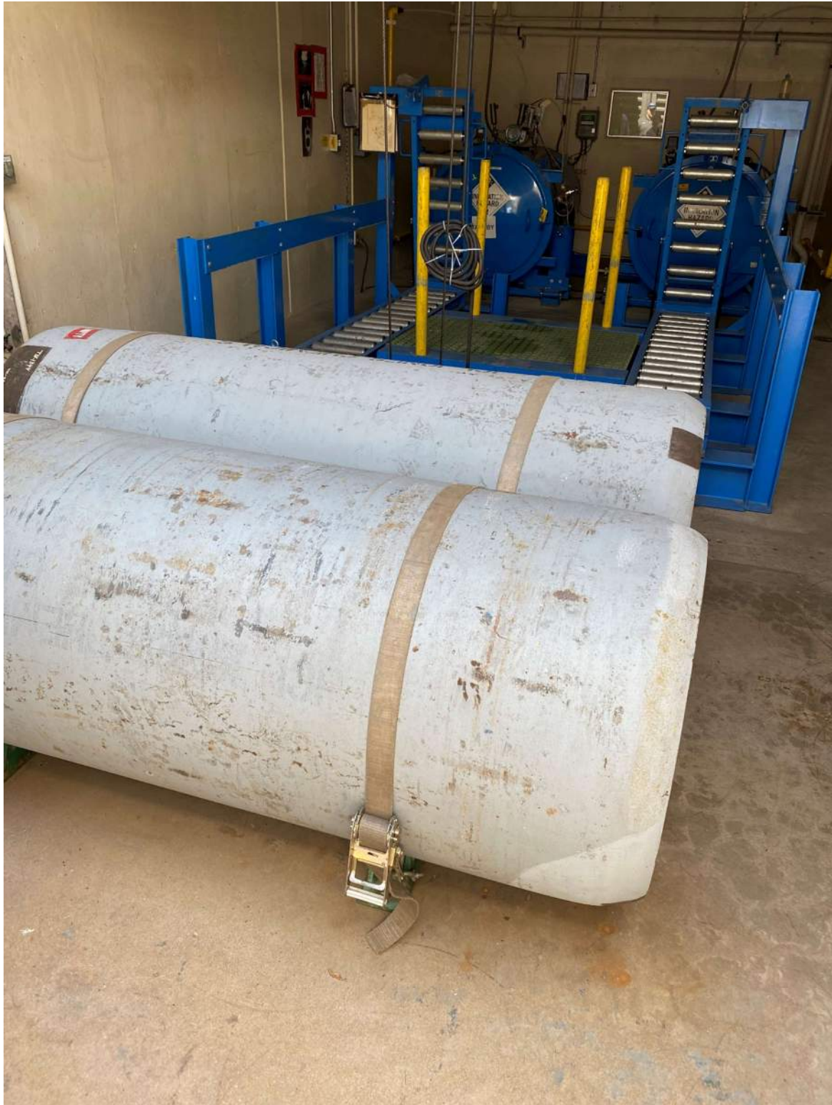
Figure 31 Chlorine Cylinders Stored Onsite
