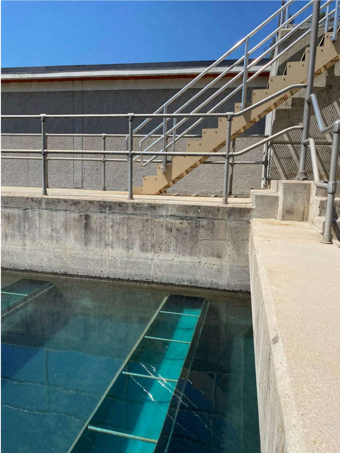
Figure 39 Filter Equipment (Seems to be in Excellent Working Condition)
