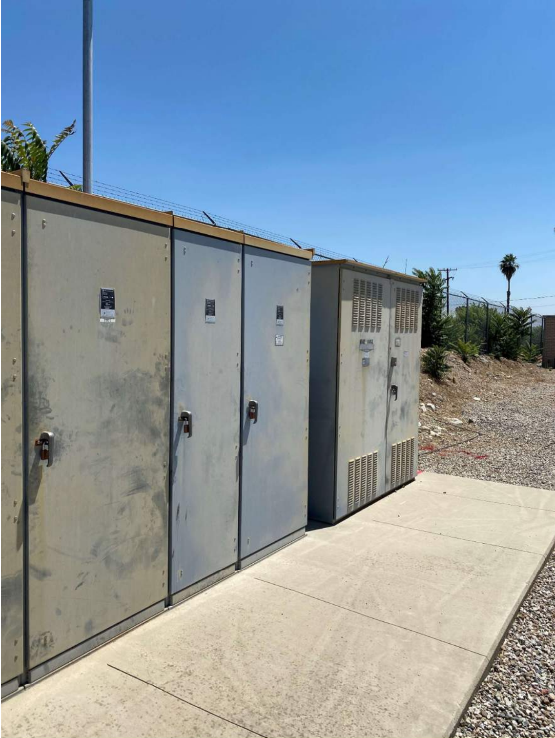
Figure 19 MCC Center for Agate Reservoir PS
