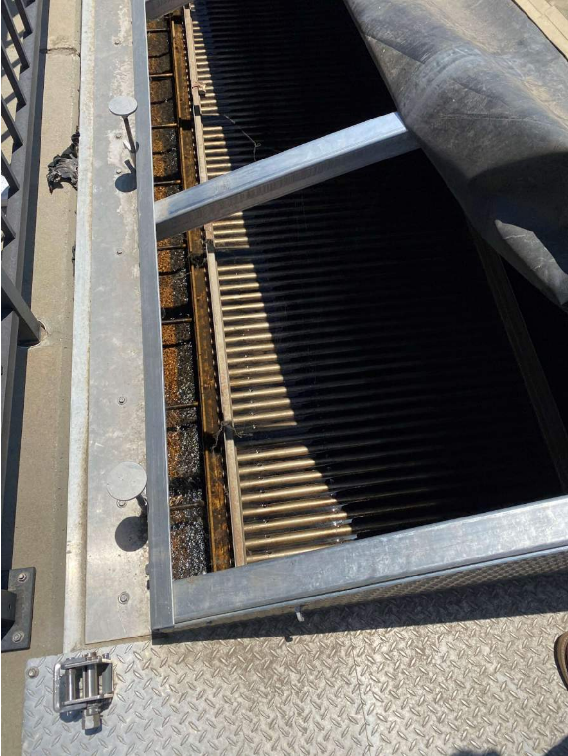
Figure 9 Hinckley WTP Flocculation/Sedimentation/Settling
