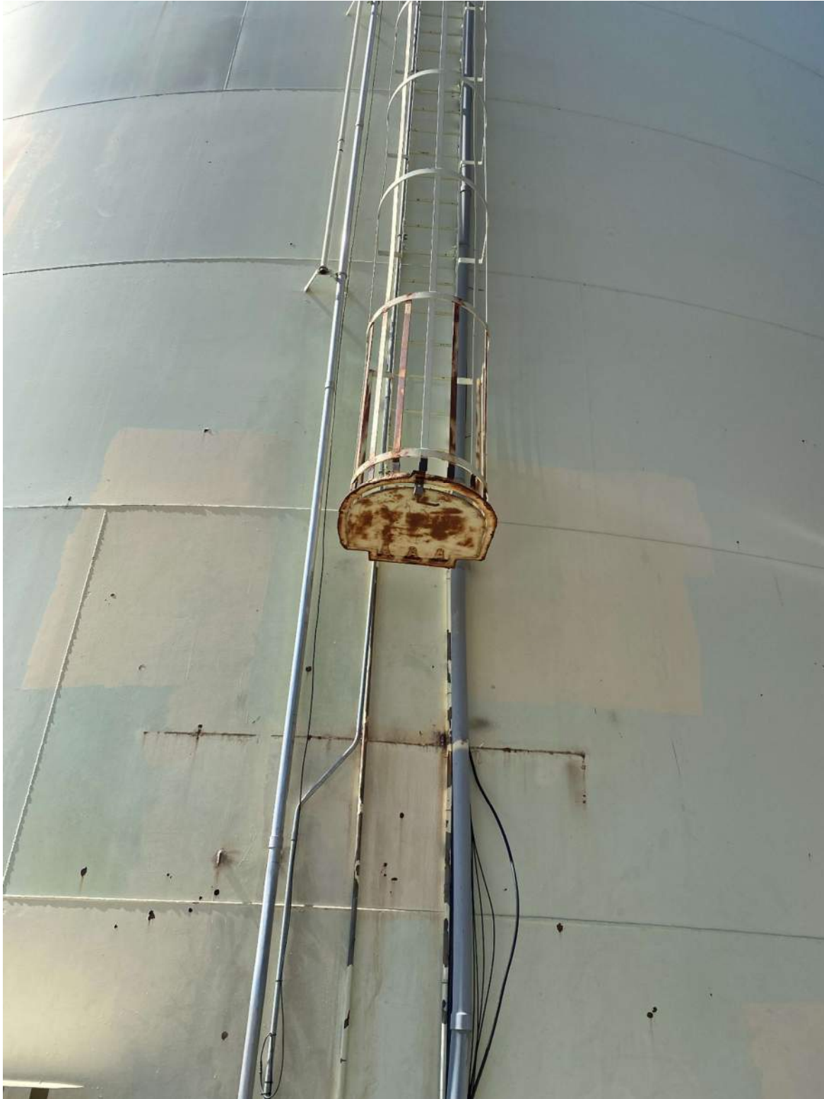
Figure 43 Steel Shell is Spot Corroded-Attached Ladders are Rusted Beyond Repair
