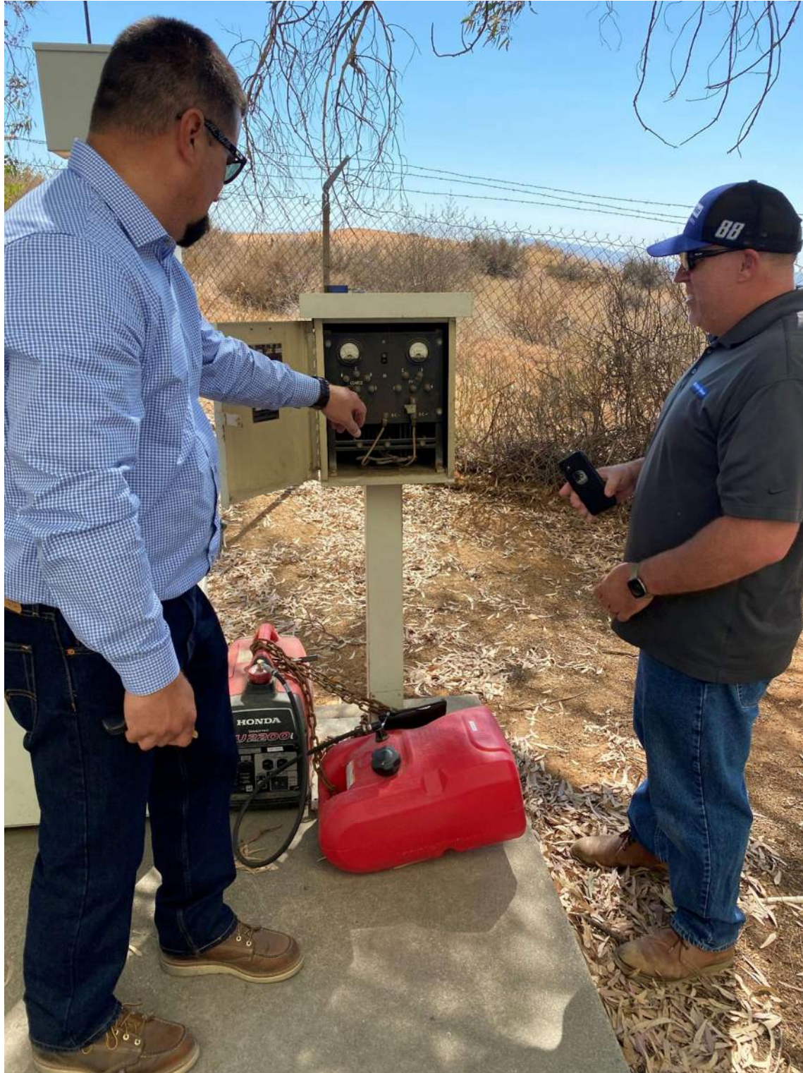
Figure 44 Reservoir Corrosion Protection Cabinet (seems antiquated)
