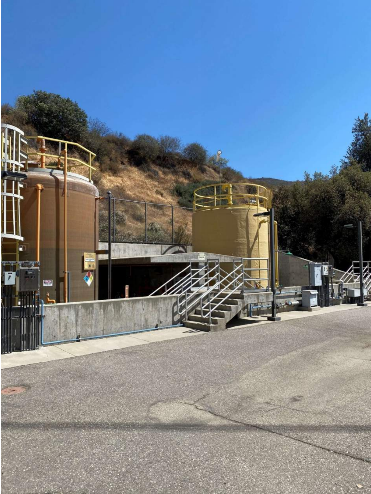
Figure 35 Chemical Storage Area with Concrete Containment-In Good Working Condition
