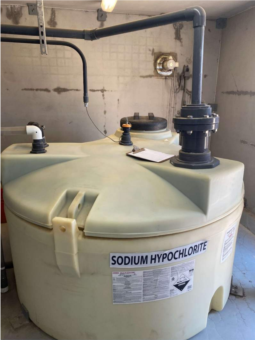
Figure 21 Disinfectant Storage at Agate Site
