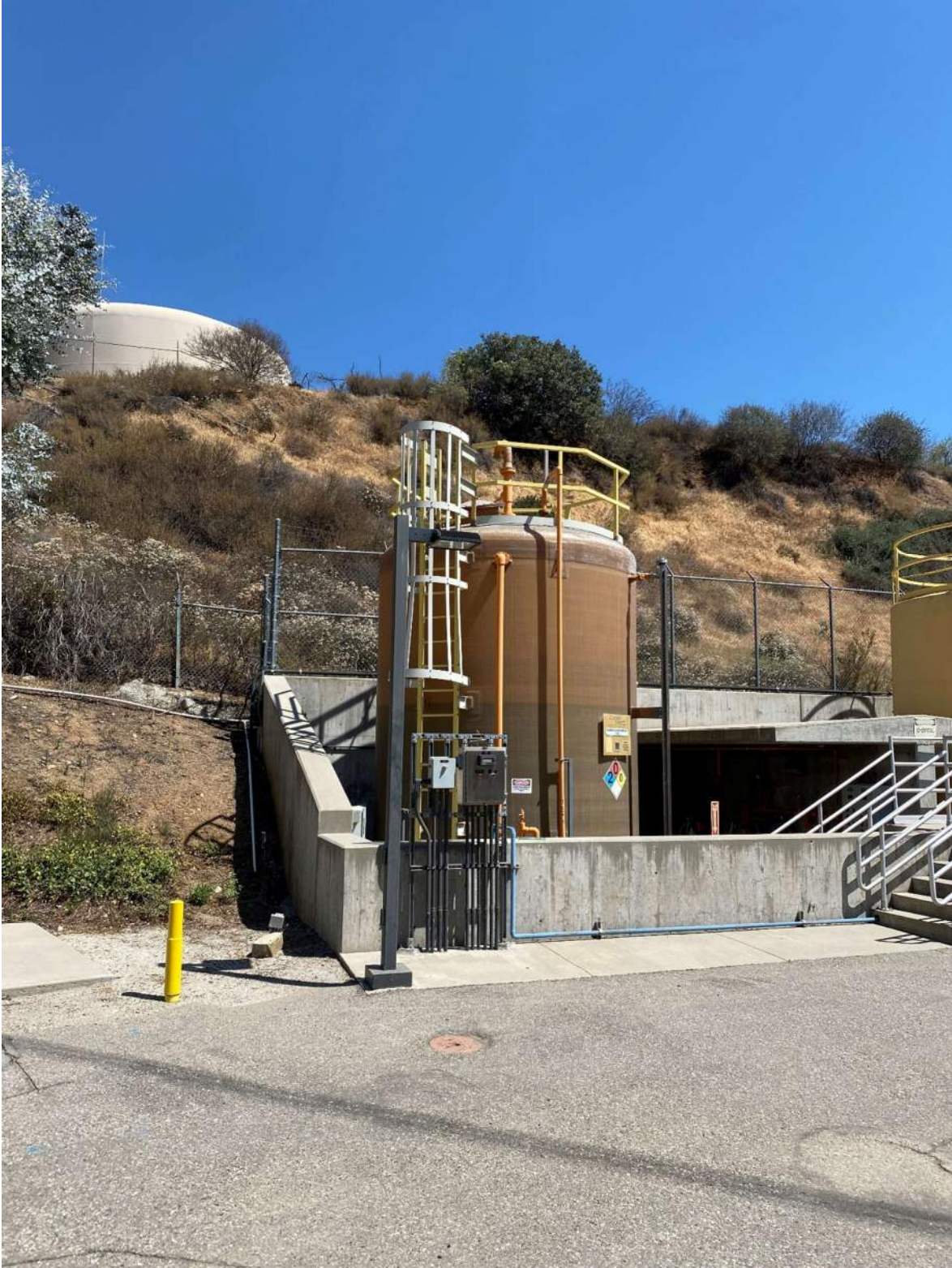
Figure 34 Effluent Reservoir Onsite
