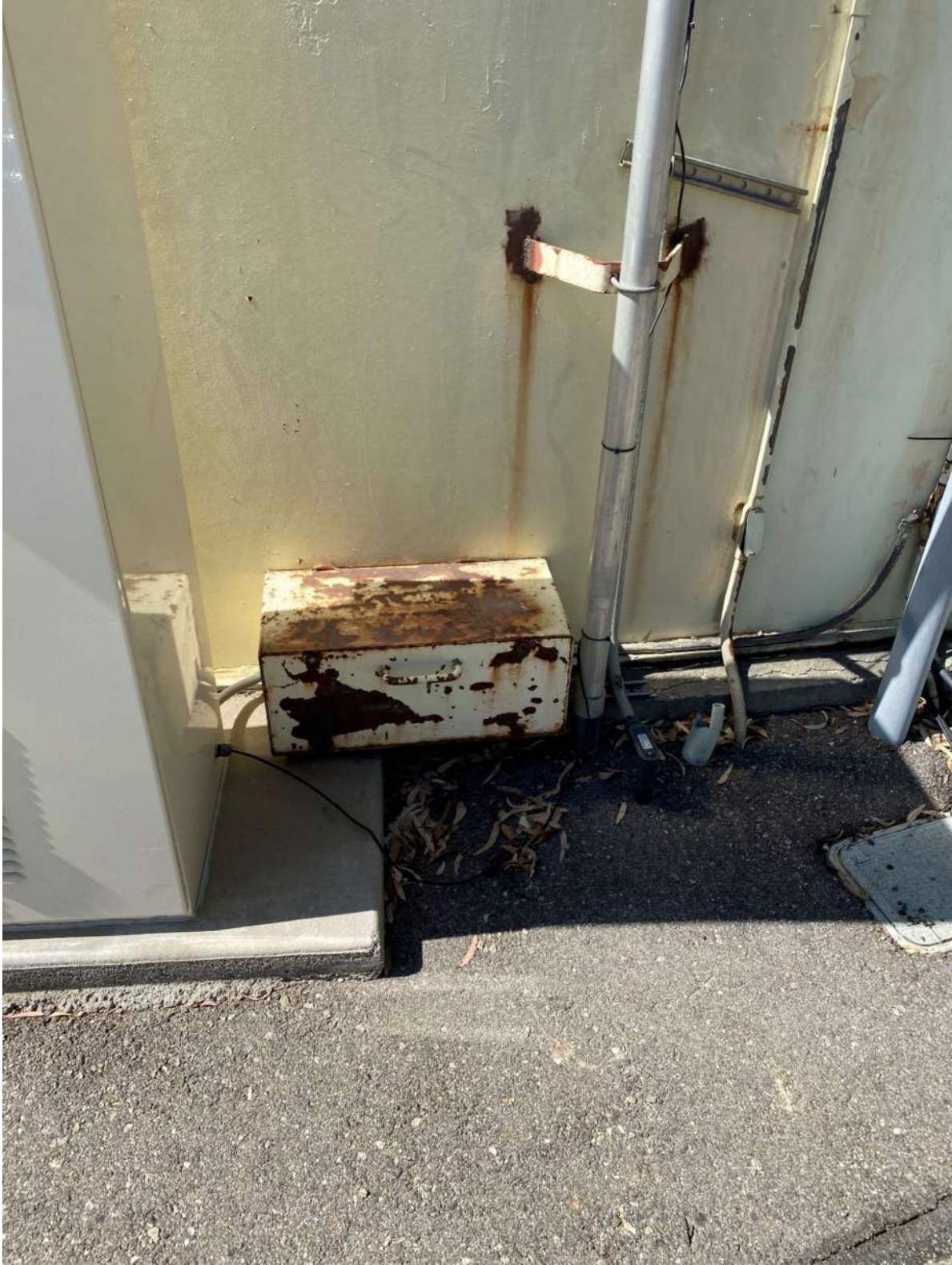
Figure 45 Close-Up of Corrosion Detail
