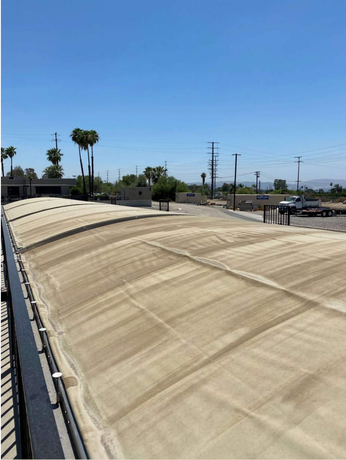
Figure 8 Hinckley WTP Flocculation/Sedimentation/Settling
