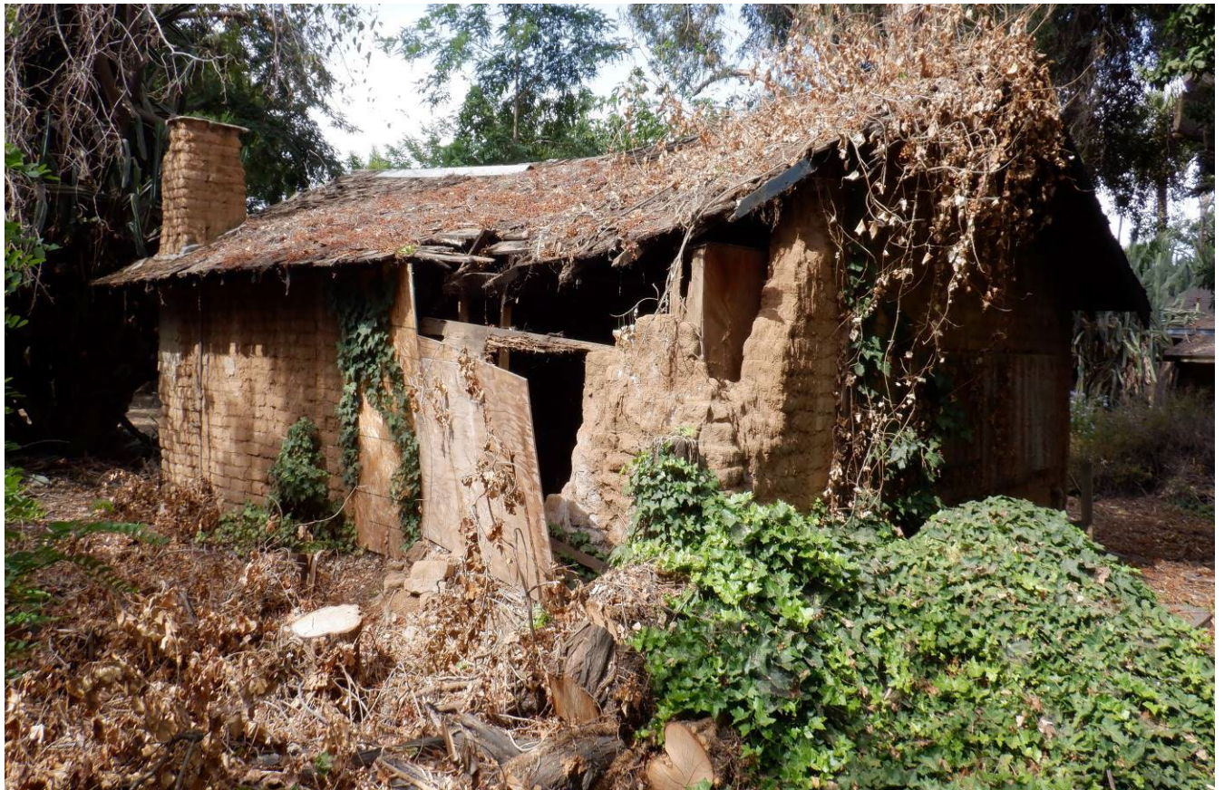
North and east elevations of c. 1925 adobe building. View southwest. (Michael Baker International, June 22, 2022)
