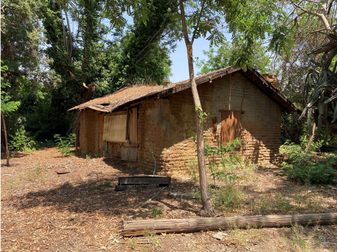
C. 1925 Adobe building. South and west elevations. View northeast. (Monte LLC, May 3, 2022)
