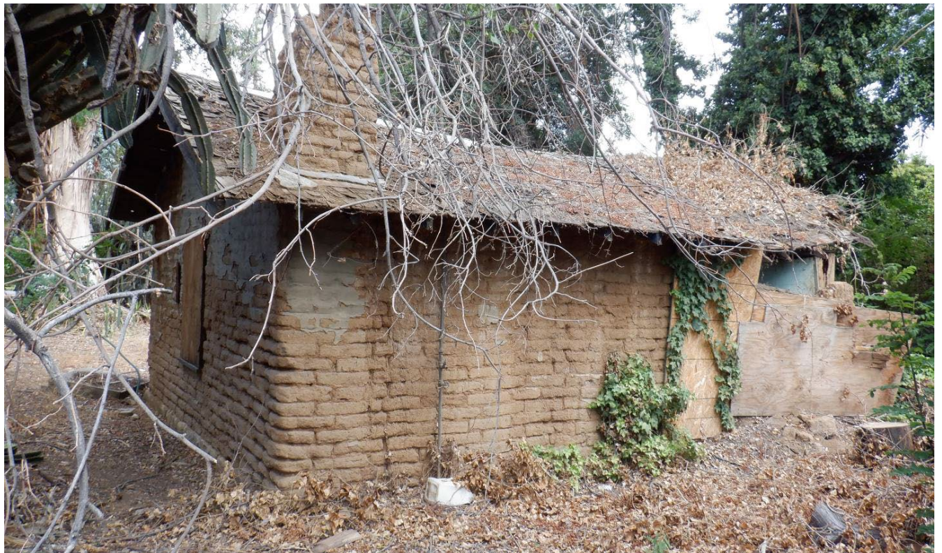
South and east elevations of c. 1925 adobe building. View northwest. (Michael Baker International, June 22, 2022)
