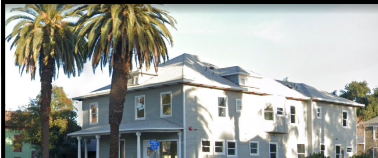
A single-family home at Olive Avenue and Grant Street undergoes a conversion to an 8-unit apartment building while also undergoing rehabilitation consistent with Secretary of the Interior guidelines for historic preservation.
