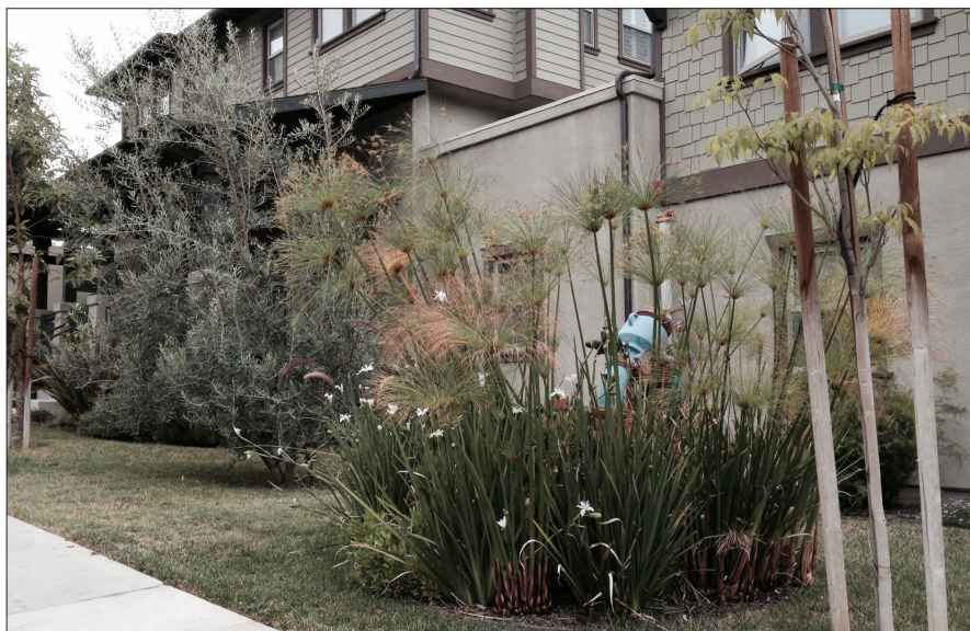
A back flow preventer that is located immediately adjacent to the building and is screened from the view of the sidewalk and street by shrubs.
