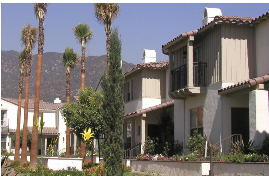
A multi-family building clad in plaster and fiber-cement siding. The vertical transition between the plaster and siding occurs at the inside corners.
