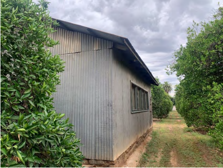
Photograph 2: Northwest elevation of the garage with the northeast elevation majorly obscured by overgrown bushes, camera facing west, July 25, 2019.
