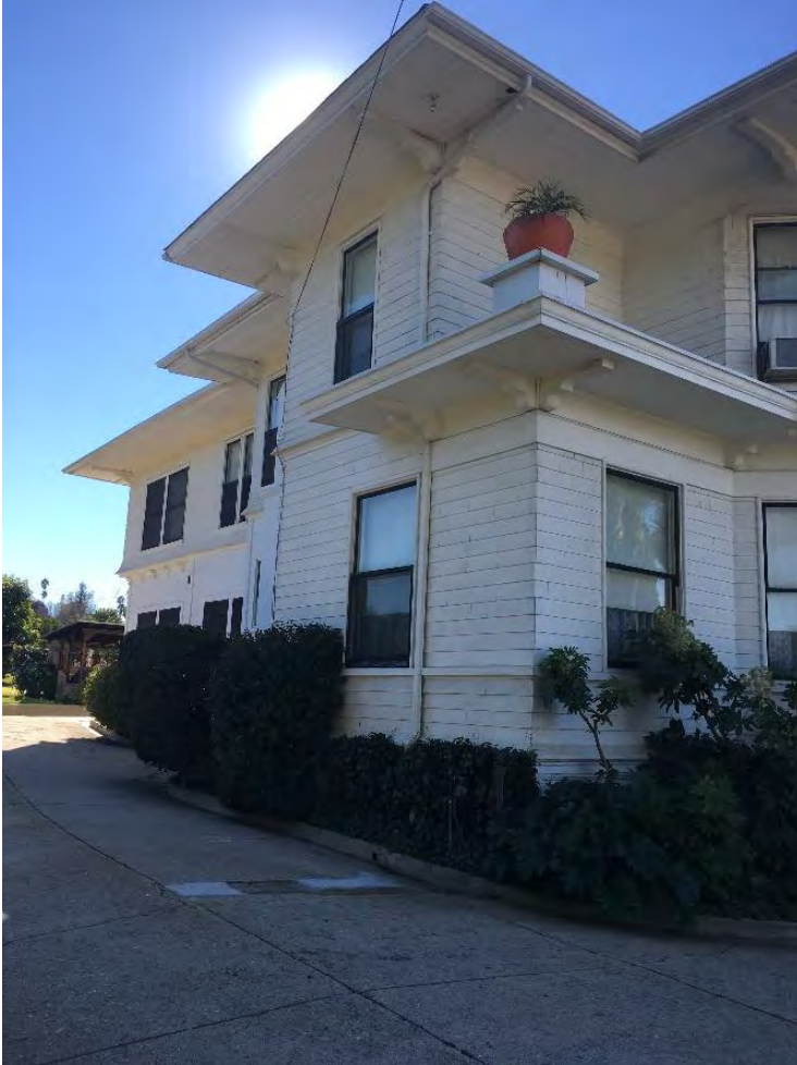
Photograph 5: Detail, windows and siding along the northeastern elevation of the residence, camera facing south, January 9, 2019.
