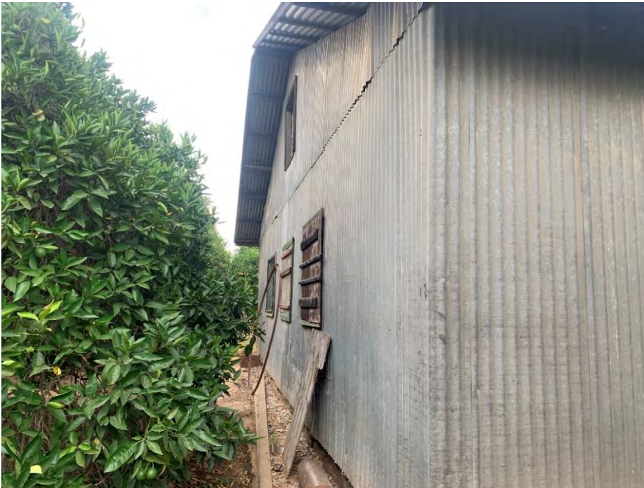
Photograph 3: View of rear northeast elevation of the garage, rear windows covered by wooden boards, camera facing southeast, July 25, 2019.
