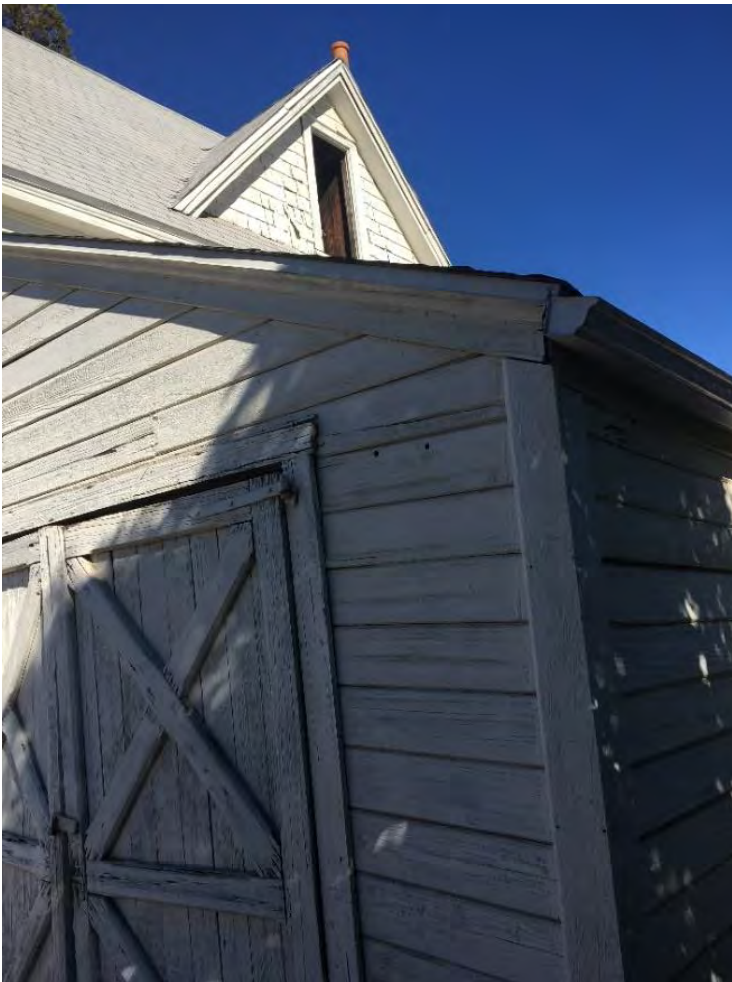
Photograph 3: Detail, close-up view of wooden siding and doors attached to southernmost corner; upstairs window of carriage house apartment also visible, January 9, 2019.
