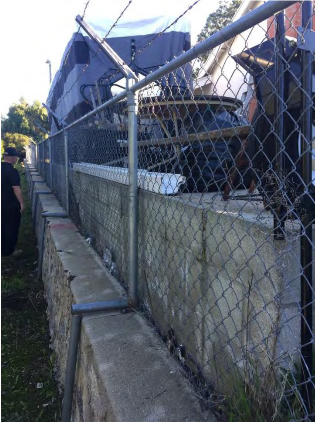
Photograph 4: View of the footing along the southeast property boundary separating it from a neighboring residence, camera facing northeast, January 28, 2020.
