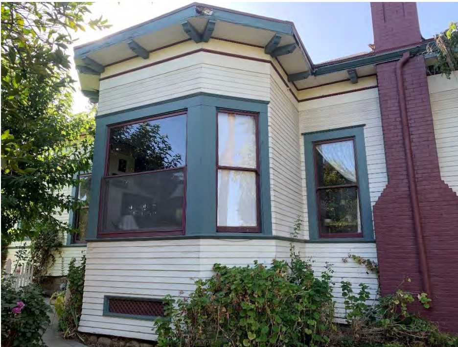
Photograph 5: Detail, second bay window adjacent to channeled brickwork chimney along northwest elevation, August 22, 2019.
