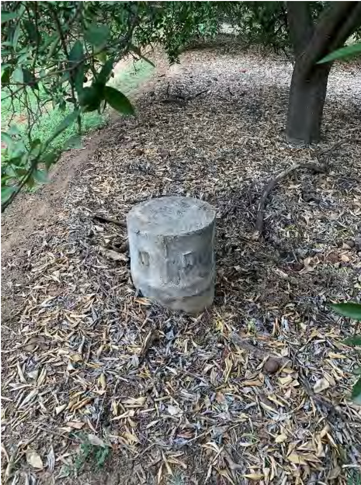
Photograph 5: Detail, a shortened standpipe used for irrigation purposes and located throughout the subject property's orange groves, July 25, 2019.
