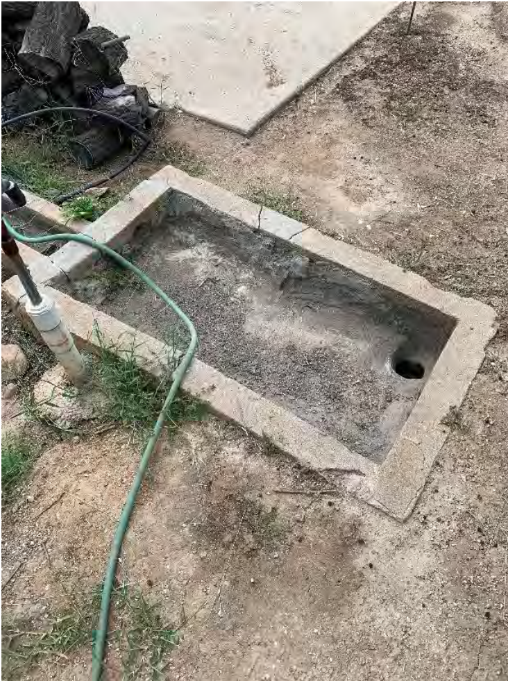
Photograph 4: Detail, alternative view of the concrete basin with small drain located in one corner, July 25, 2019.
