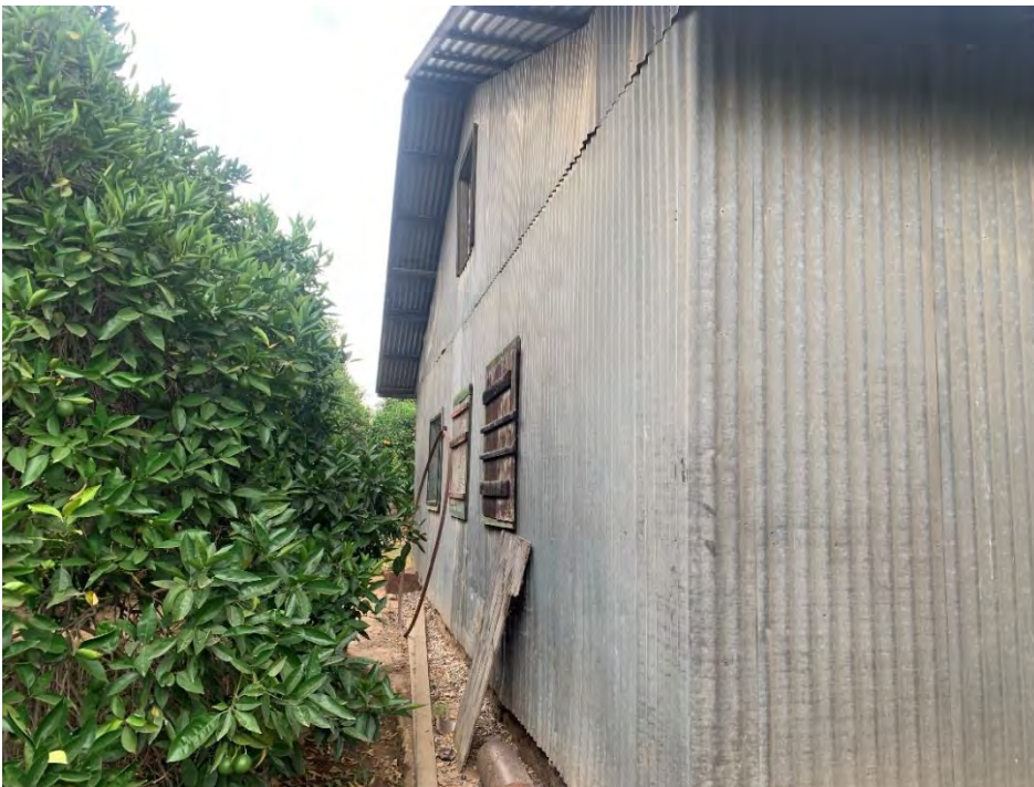
Photograph 3: View of rear northeast elevation of the garage, rear windows covered by wooden boards, camera facing southeast, July 25, 2019.
