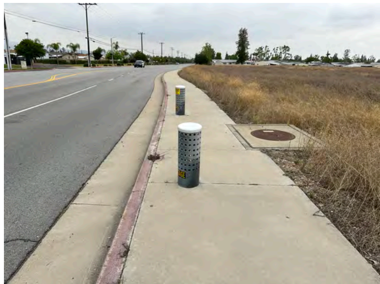
Transformer Vault on SE Corner of Site
