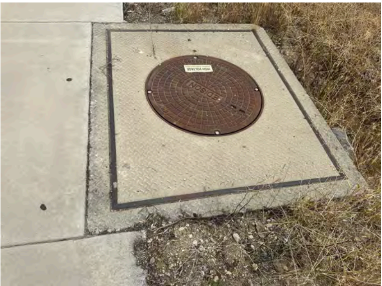
Transformer Vault on SE Corner of Site
