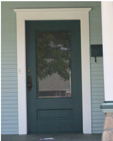
Single wood doors with paneling and glazing are common features of pre-war houses in Redlands.
