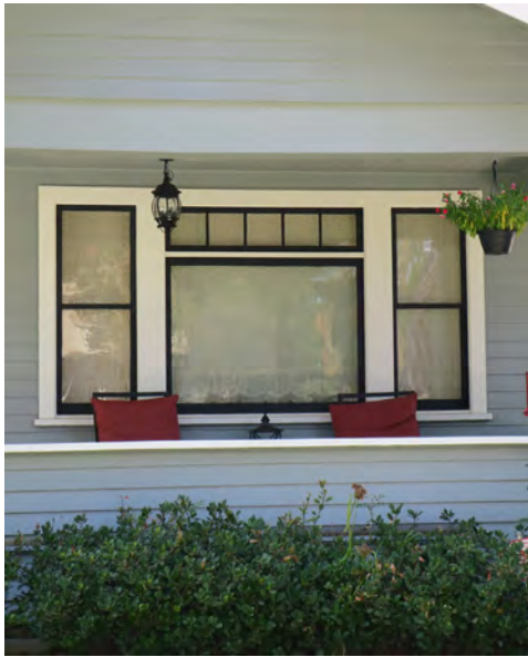
Vertically oriented, double-hung wood windows are typical of houses in the city's pre-war neighborhoods.
