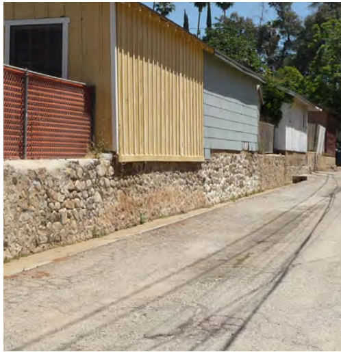
Arroyo stone foundations are an important architectural feature of many historic houses in Redlands and should be preserved.
