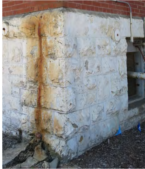
A cast stone foundation that is in need of repair.
